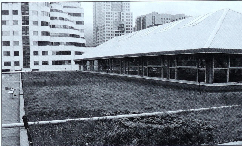
Green roofs can store storm waters
